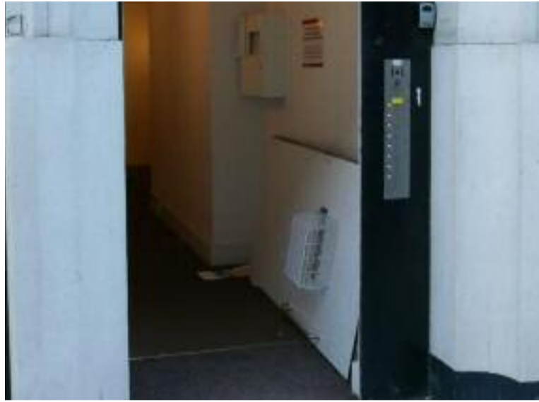
Front door was broken and left open for weeks.
